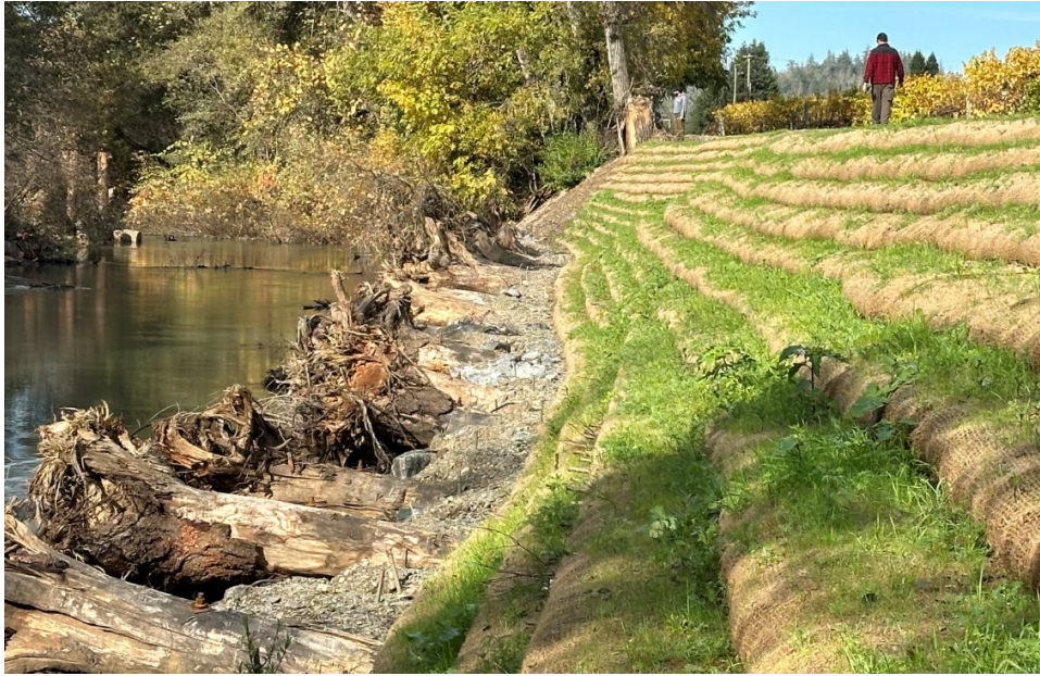
Photograph taken November 21, 2023 of the upstream end of a completed Reach 10 biotechnical bank repair.
