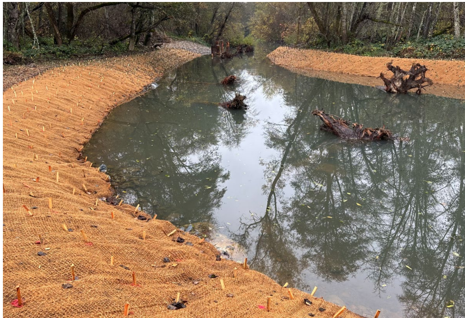
Photograph taken on 12/7/23 showing nearly completed section of new side-channel habitat feature at site 4C.
