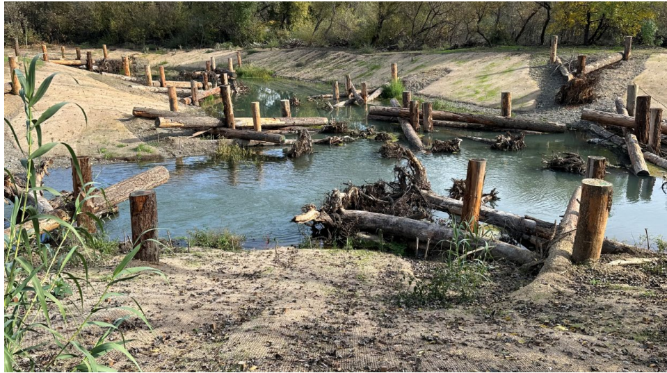
Photograph taken November 21, 2023 of an alcove in the site 10A2 Side Channel.
