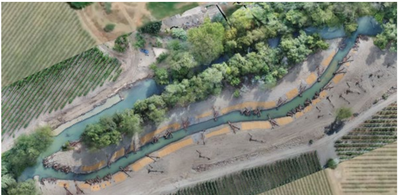
Post-construction drone photo of reach 13 enhancement reach (Pedroncelli) in Dry Creek. Photo taken September 6, 2023.
