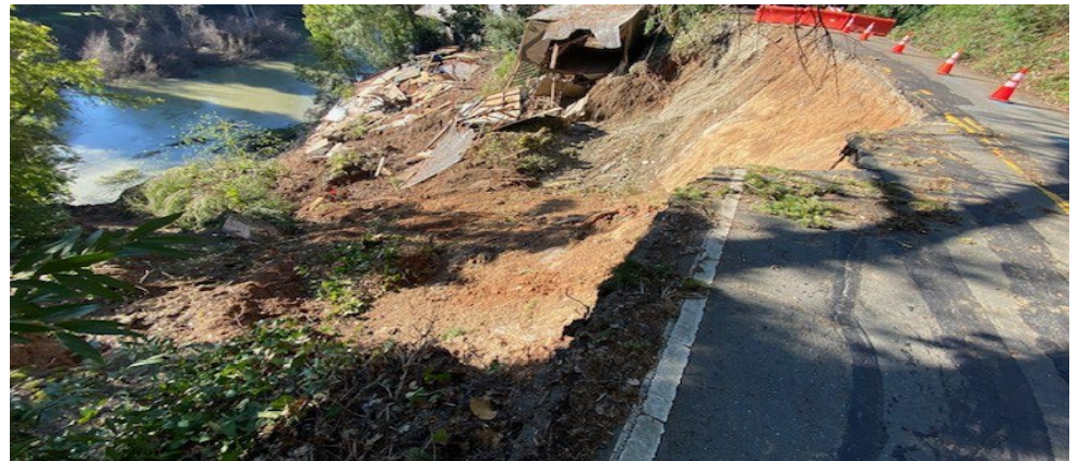
Westside Road Landslide at River Road
