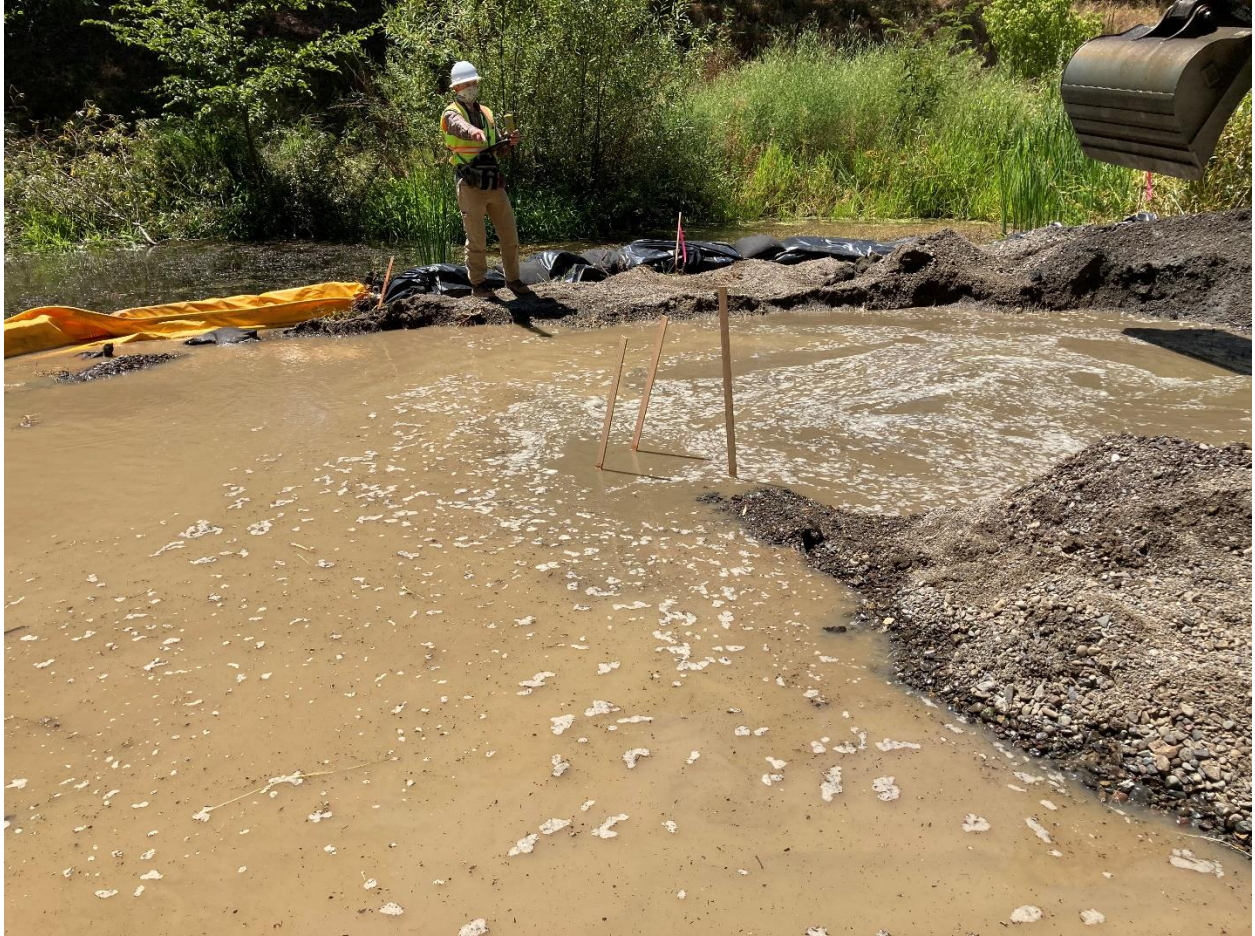
Photo 5.1.29. Reach 7 - Van Alyea Site. Removal of gravel material and locating freshwater conduit outlet in process. July 30, 2020.
