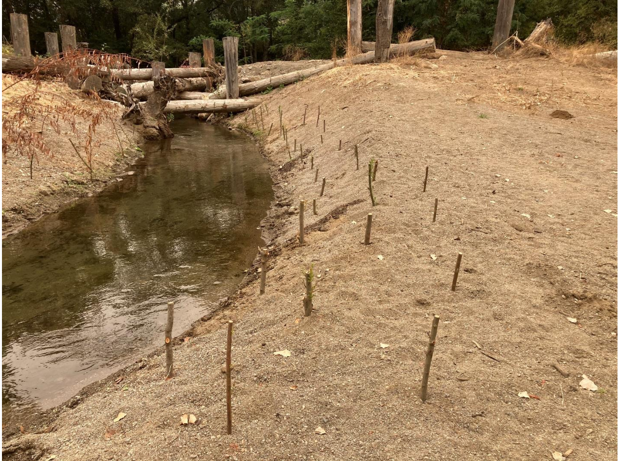
Photo 5.1.37. Reach 8 - Carlson Site. New willow cuttings sprouting along inlet area that was cleared. September 10, 2020.
