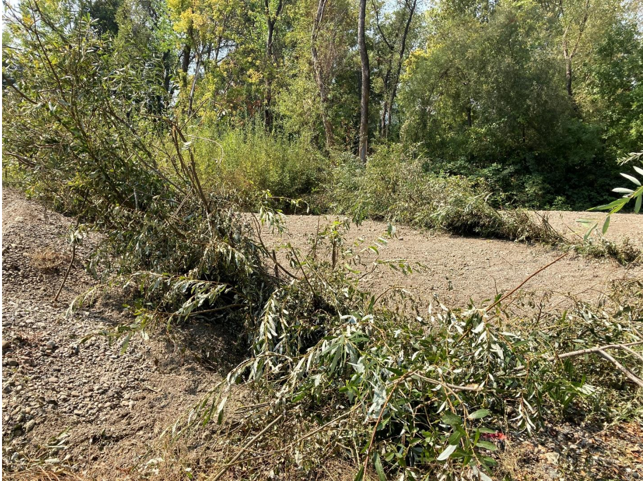
Photo 5.1.19. Reach 4A. New willow baffles installed to discourage paths for future aggradation within the habitat site. September 21, 2020.
