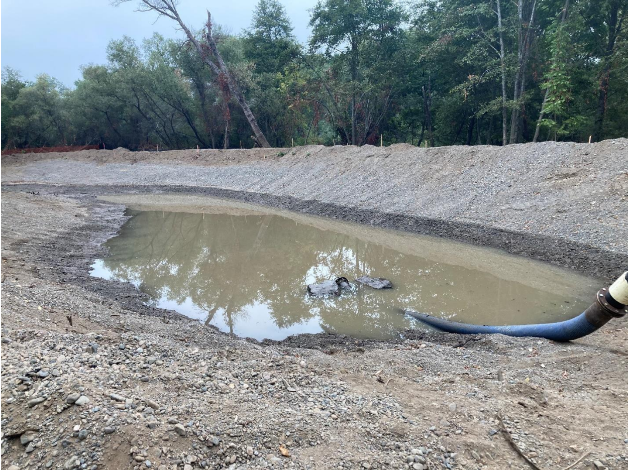
Photo 5.1.5. Phase 3, Part 3. Initial clearing of habitat site work area and being used as a dewatering basin for the bank stabilization work. September 10, 2020.
