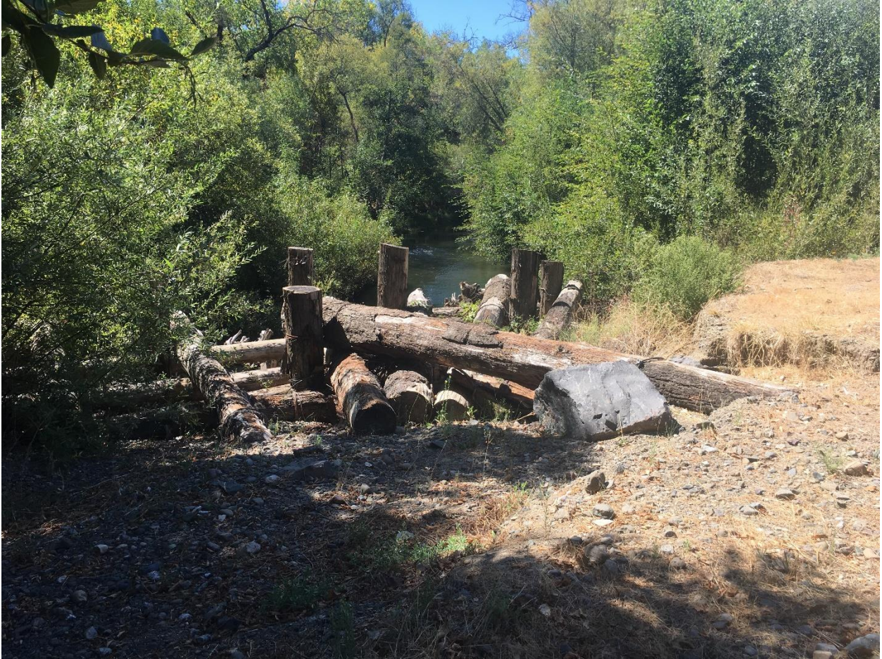
Photo 5.1.21. Reach 7 - Farrow site. Photo shows eroded area exposing back portion of engineered logjam at outlet of backwater pond. September 13, 2018.
