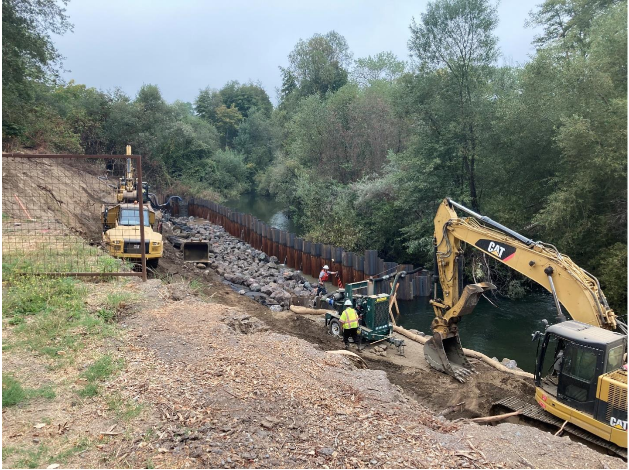
Photo 5.1.4. Phase 3, Part 3. Rock slope protection construction in progress. Note sheet-pile isolating work area from active flow of Dry Creek. September 10, 2020.
