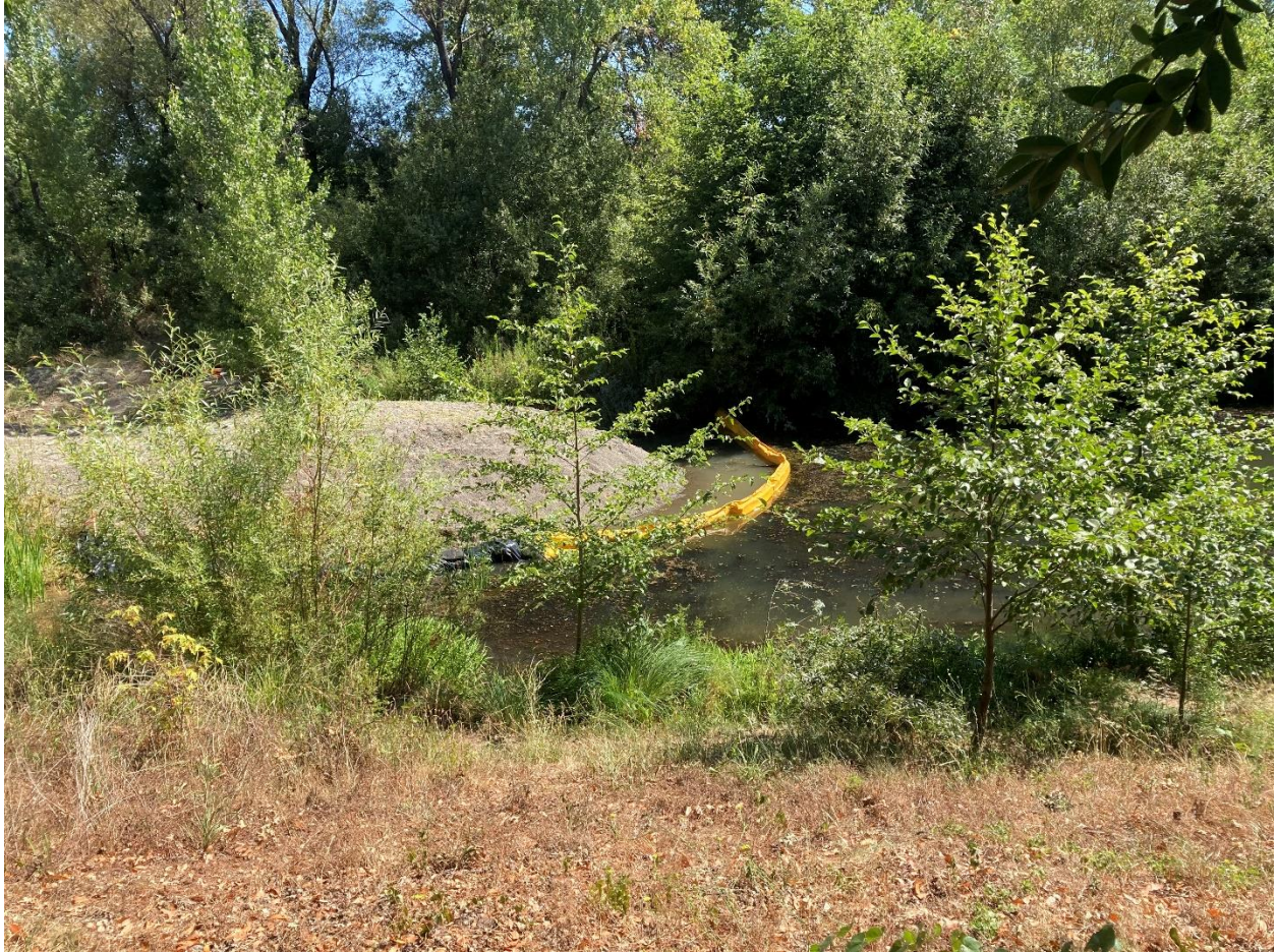
Photo 5.1.28. Reach 7 - Van Alyea Site. Gravel deposited in upper end of backwater pond, covering outlet of freshwater conduit from Dry Creek. Photo shows turbidity curtain installed around work site prior to removing gravel. July 29, 2020.
