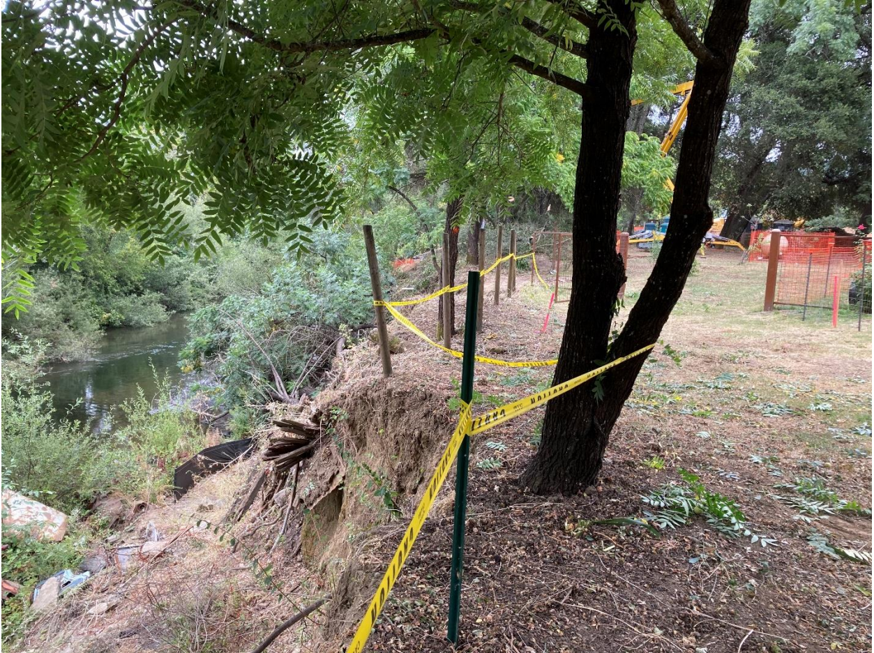
Photo 5.1.1. Phase 3, Part 3. Upper end of bank stabilization work area, looking downstream pre-project condition. July 30, 2020.
