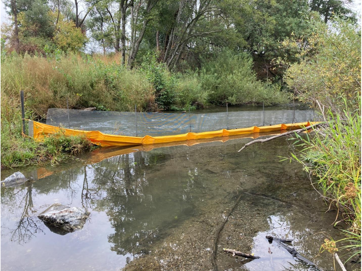
Photo 5.1.15. Reach 4A. Turbidity curtain and fish screening installed at downstream end of habitat work. September 3, 2020.
