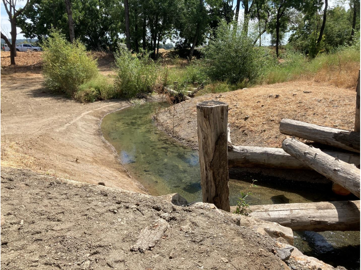
Photo 5.1.35. Reach 8 - Carlson Site. Photo showing inlet to the side-channel cleared of sediment blocking flow. August 18, 2020.
