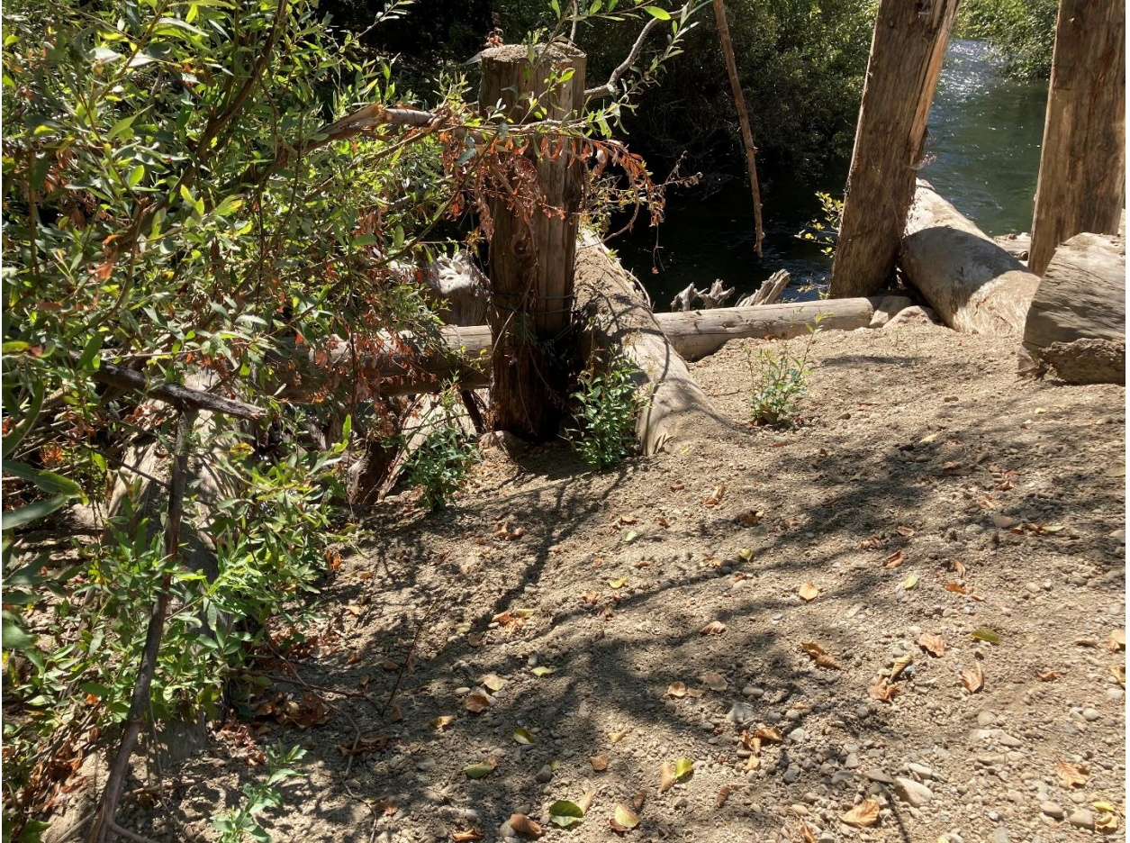
Photo 5.1.24. Reach 7 - Farrow site. New growth on willow cuttings at engineered logjam. September 17, 2020.
