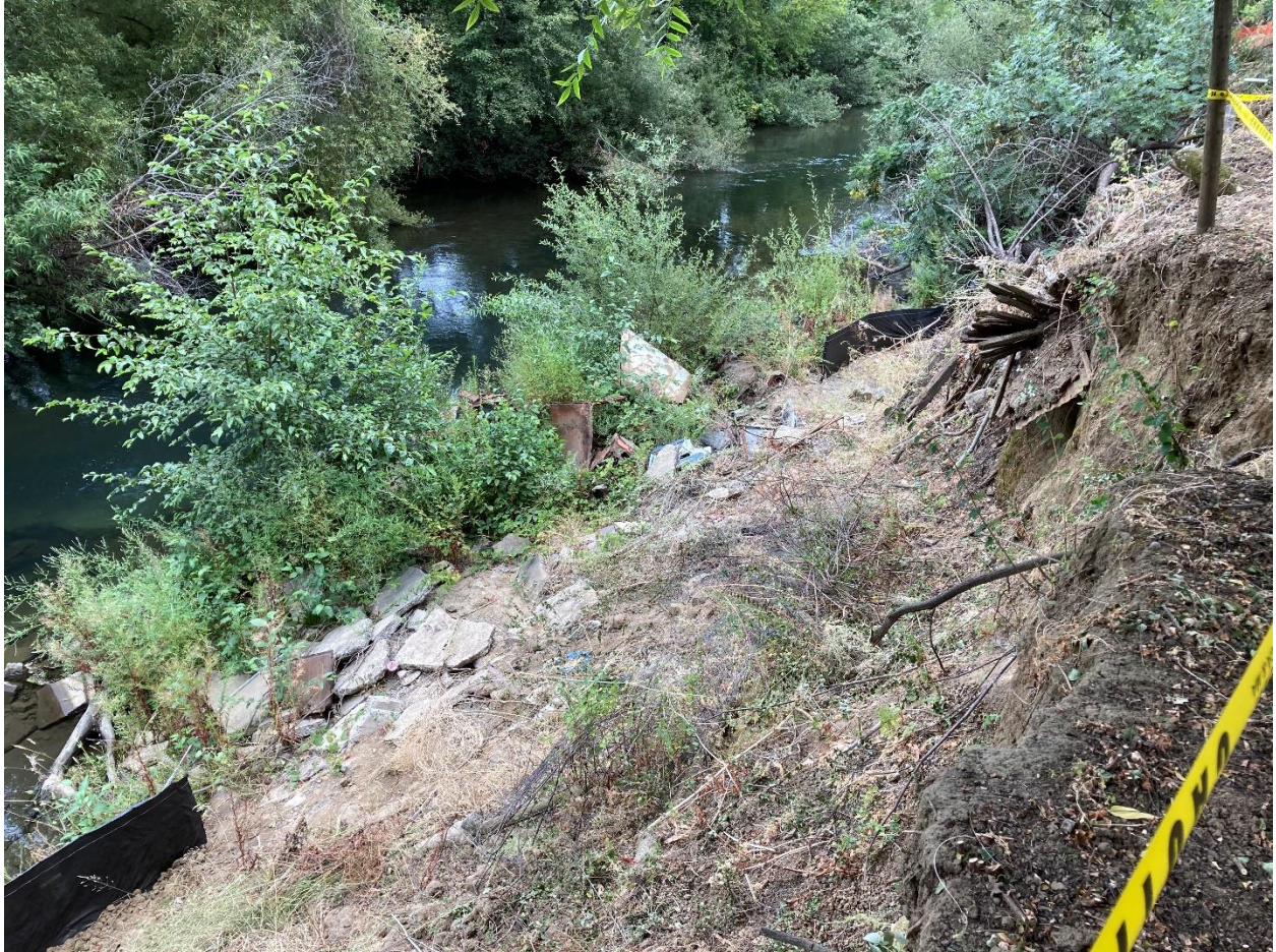
Photo 5.1 2. Phase 3, Part 3. Upper end of bank stabilization work area, looking downstream pre-project condition. July 30, 2020.
