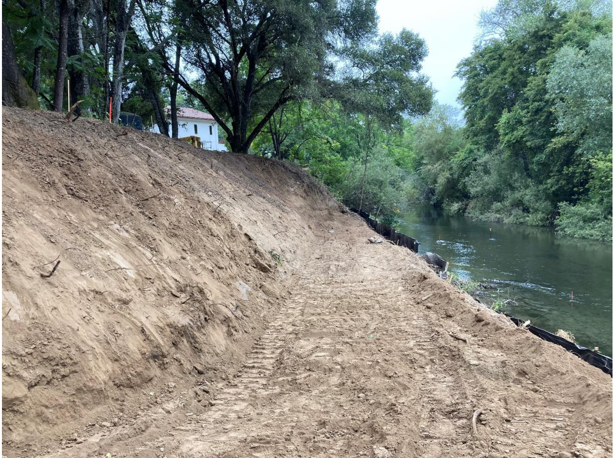
Photo 5.1.3. Phase 3, Part 3. Lower end of bank stabilization work area, looking upstream. Initial clearing and access road underway. July 30, 2020.
