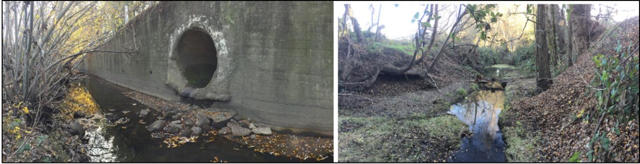
Figure 12. Concrete retaining wall with 48" stormdrain outlet on opposite bank from the Penngrove Community Park (left) and typical channel near the downstream end of the baseball field in the park (right).
