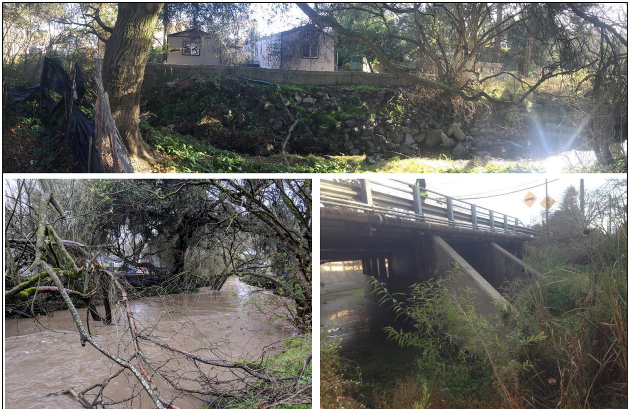
Figure 10. Photos from the Penngrove Center Reach: Penngrove Village Mobile Home Park with floodwall (top), channel during storm flows near V-Dolan yard (left) and Petaluma Hill Road bridge looking downstream (right).
