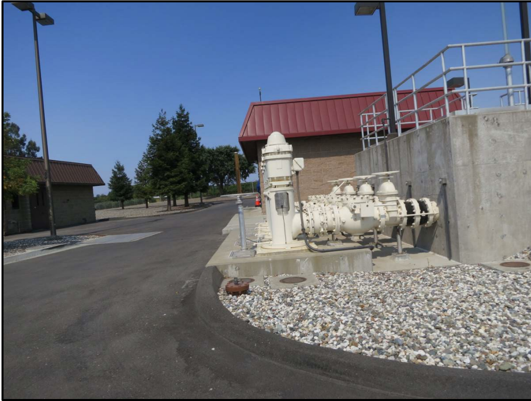
Figure 12: Flexible Connections (Source: SVCSD WWTP – September 2016)
